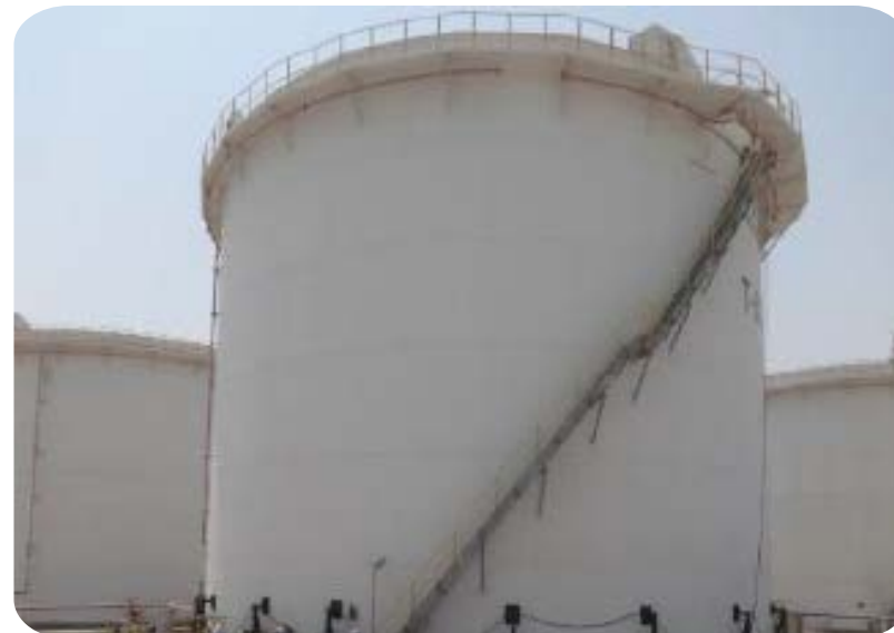
JACKING SYSTEM - STORAGE TANKS
