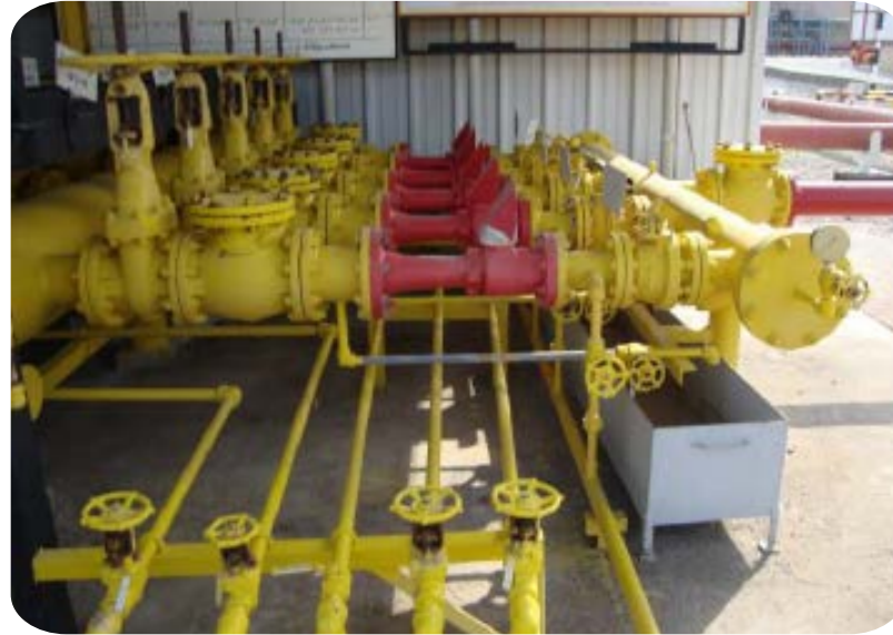
FIRE FIGHTING SYSTEM
