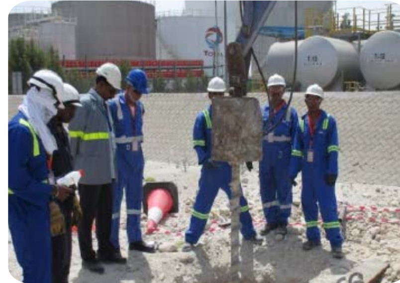
GROUND WATER MONITORING SYSTEM
