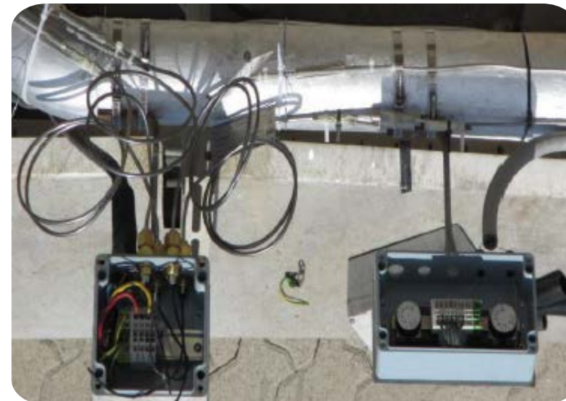
ELECTRICAL HEAT TRACING SYSTEM
