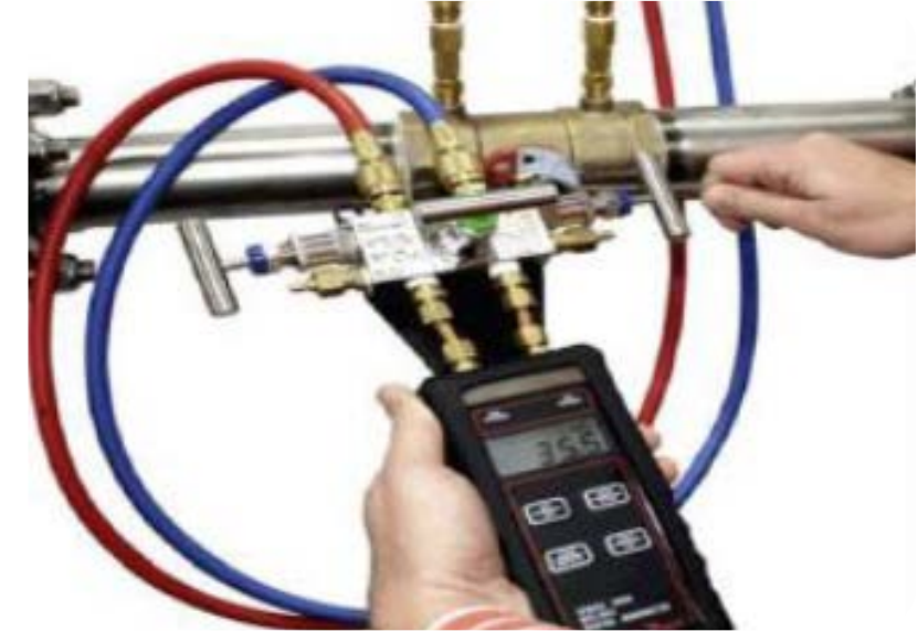
AIR CONDITIONER WORK WITH MEP
